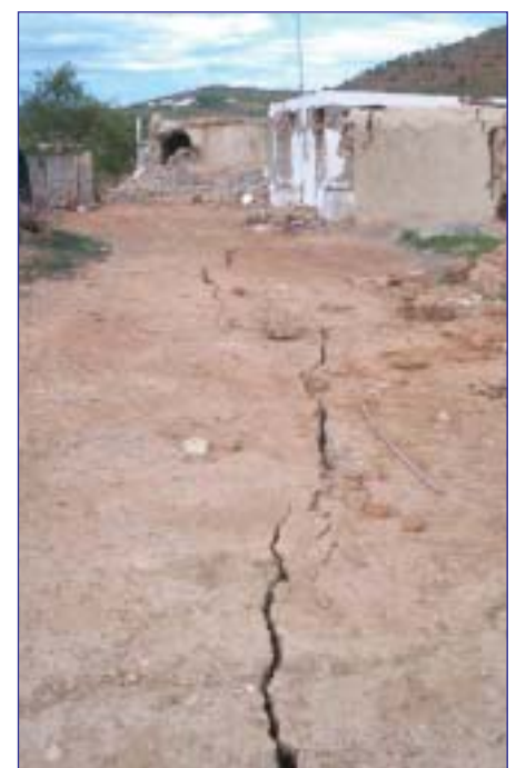
Figure 2: N050° oriented fissures in the Ait Kamra area.
